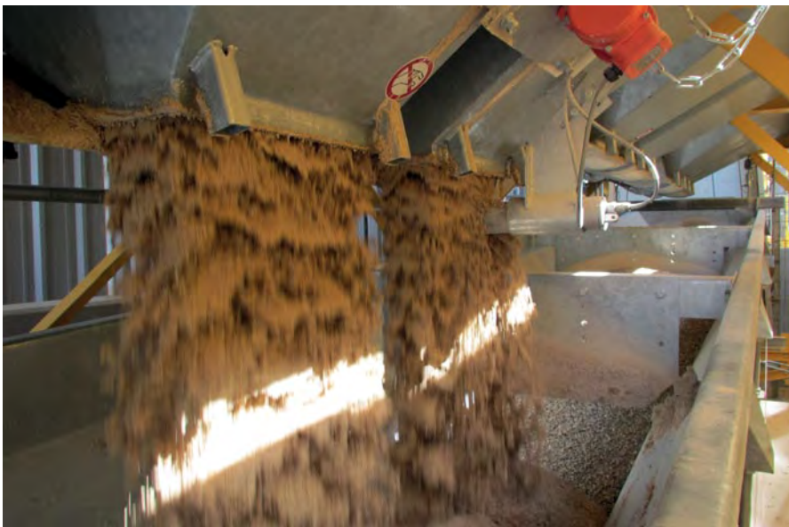
Figure 9: Sand is batched onto the weigh belt conveyor under the four-bin aggregate storage system. ACT Hydrotester microwave probes are installed in the sand bins to accurately measure and compensate for moisture content. The MobilMat PCS Control HydroMat system automatically accounts for aggregate moisture in calculating required total water for proper W/C ratio, so critical in SCC production.
