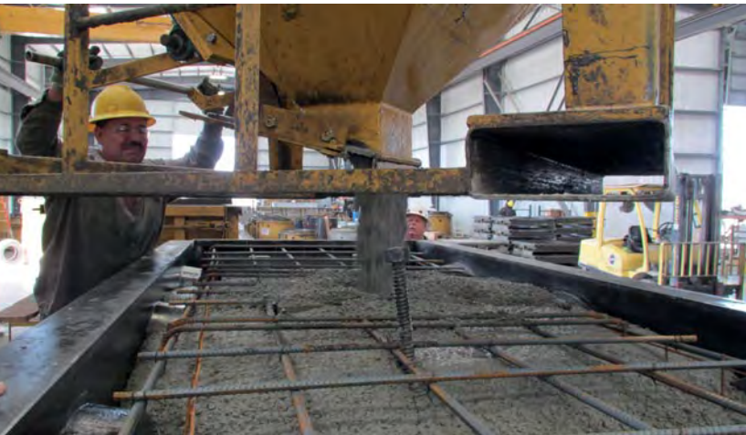
Figure 13: Crane operator Jose Gonzalez pours SCC from a crane bucket into a communication vault form. SCC is poured into a single spot on the form and allowed to flow naturally, saving time and requiring no vibration.
