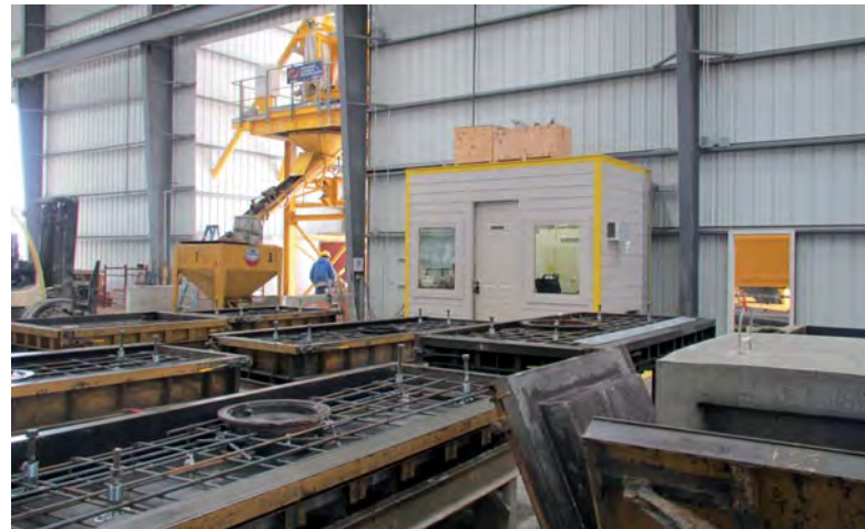
Figure 14: Centrally located ACT MobilMat batching system in background, with control room just to its right. A crane bucket stands ready to receive the next batch of SCC. Three bridge cranes are used to reach all areas of the production floor. PCS Control enables automated batching control that frees staff to focus on other plant operations.
