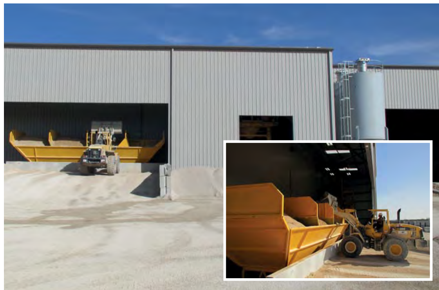
Figure 8: Capital Precast's new MobilMat batching system is installed just outside the main production facility, and enclosed for all-weather operation. Two 1,800 cu ft silos, at right, store Portland cement and fly ash, necessary for SCC production. Inset photo (lower right) a front-end loader charges the four aggregate bins with sand and stone.
