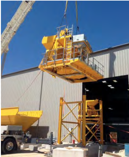
Figure 6: Modular mixer platform for new MobilMat Mo3450-4-PCS batch plant is craned into place under the direction of Ash's brother Mason Wineinger (bottom right) just outside Capital Precast's new 50,000 s.f. facility in San Marcos, TX. MobilMat plant components are pre-wired, pre-plumbed and tested at the factory and make installation and start-up smooth and fast.
